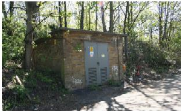
3 Existing electricity substation
